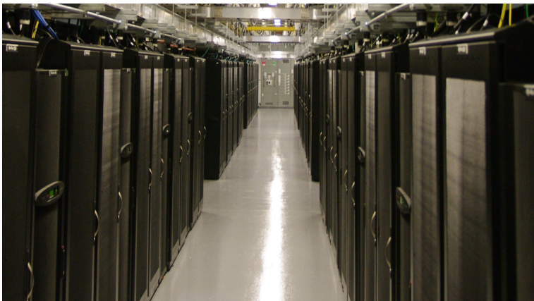
Massachusetts Green High Performance Computing Center (mghpcc.org)
